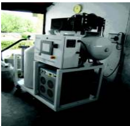
Figure 16: A small Liquid Nitrogen plant recently installed at Mt Abu Observatory at Gurushikar.
